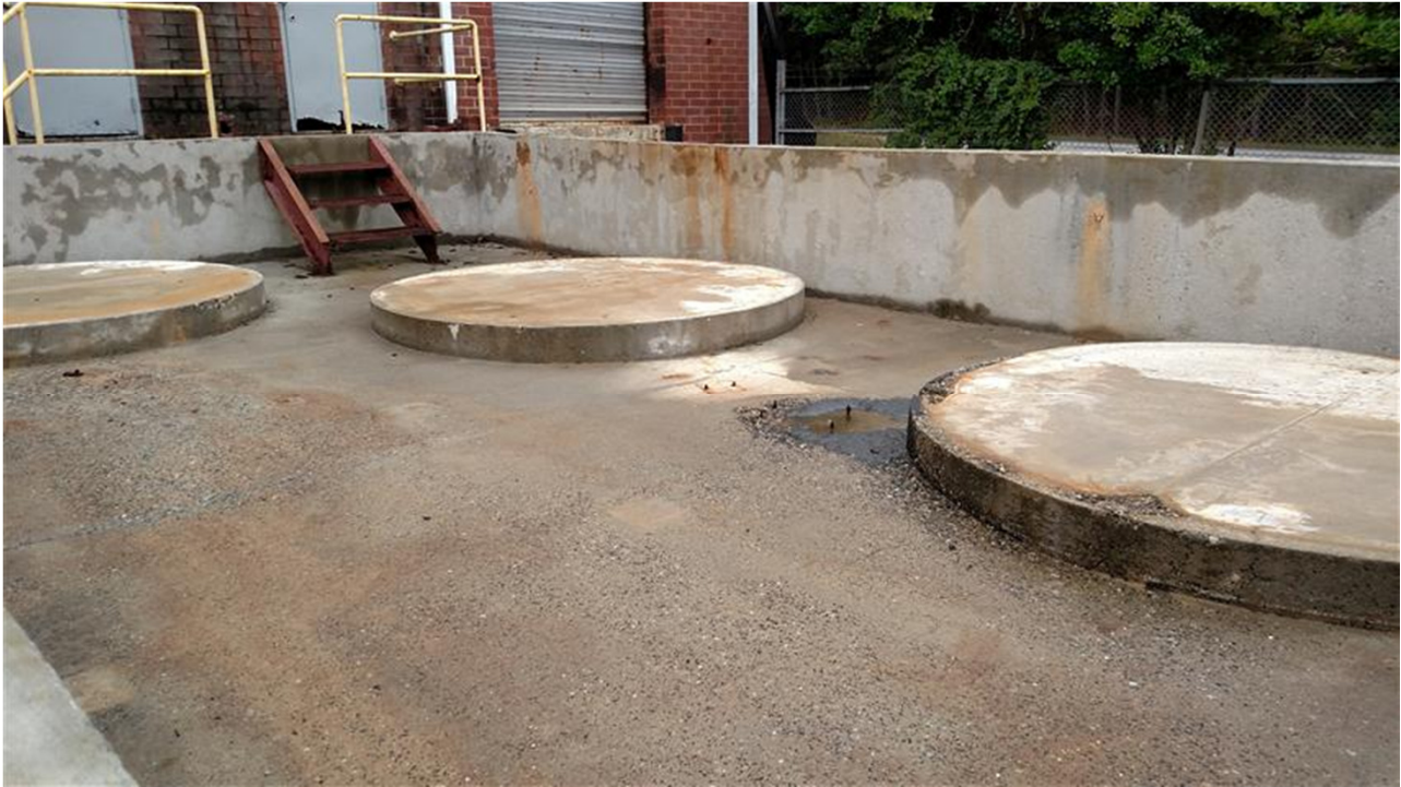
9. View of former AST secondary containment along eastern exterior wall of the project building.
