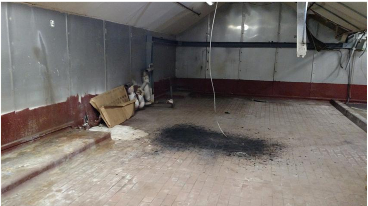
26. Corrosion, staining and floor drain in the second floor production area.
