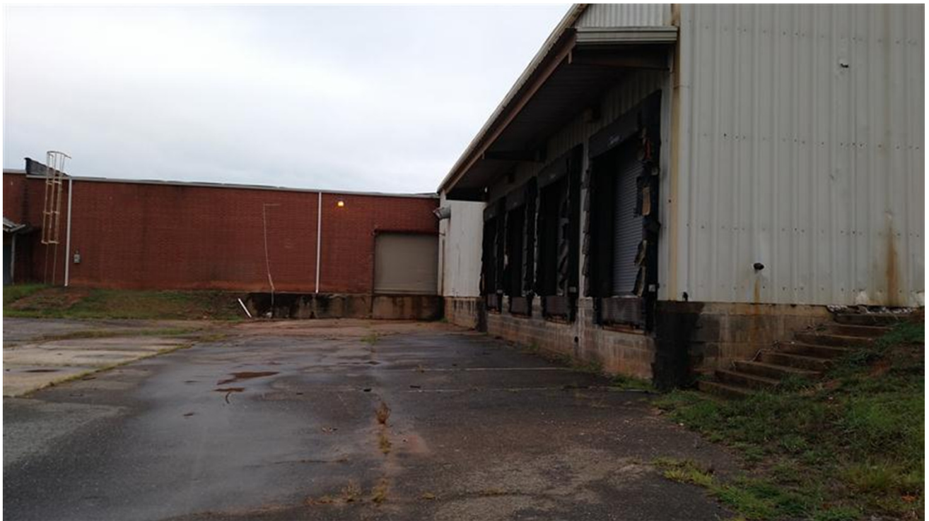
6. Loading dock area along the southern exterior wall of the project building.
