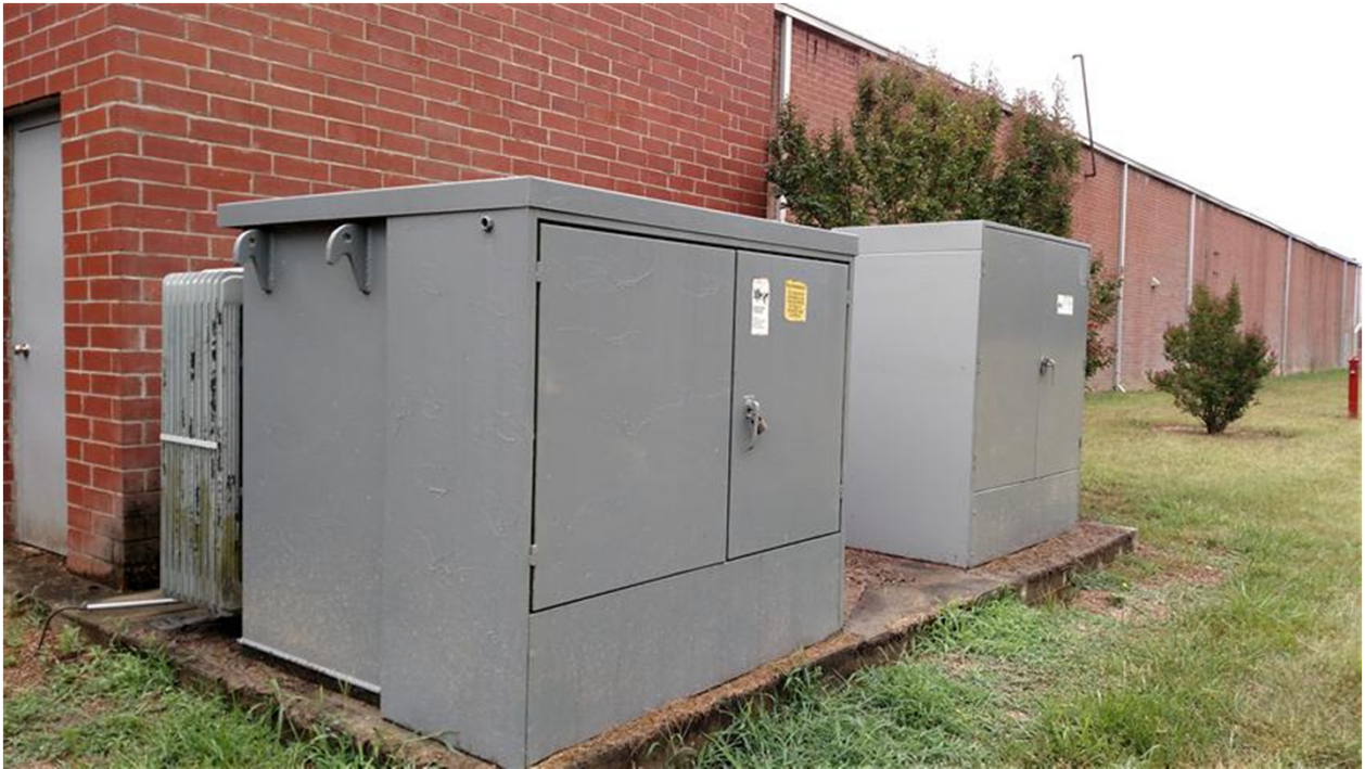
13. View of pad-mounted transformers located along the northern exterior wall of the project building and labeled as PCB containing.
