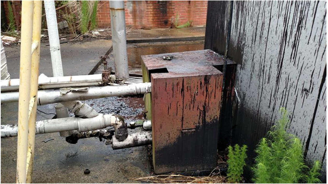
11. Staining on the #6 fuel oil AST.
