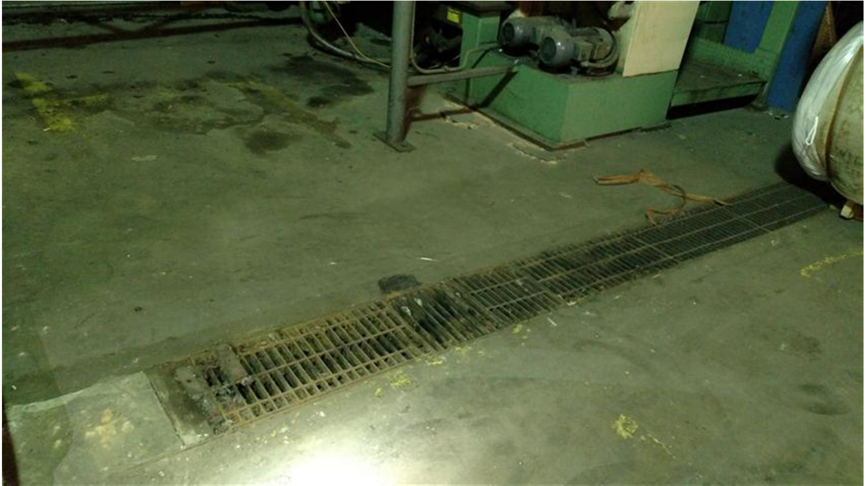
17. Floor drains in finishing area.
