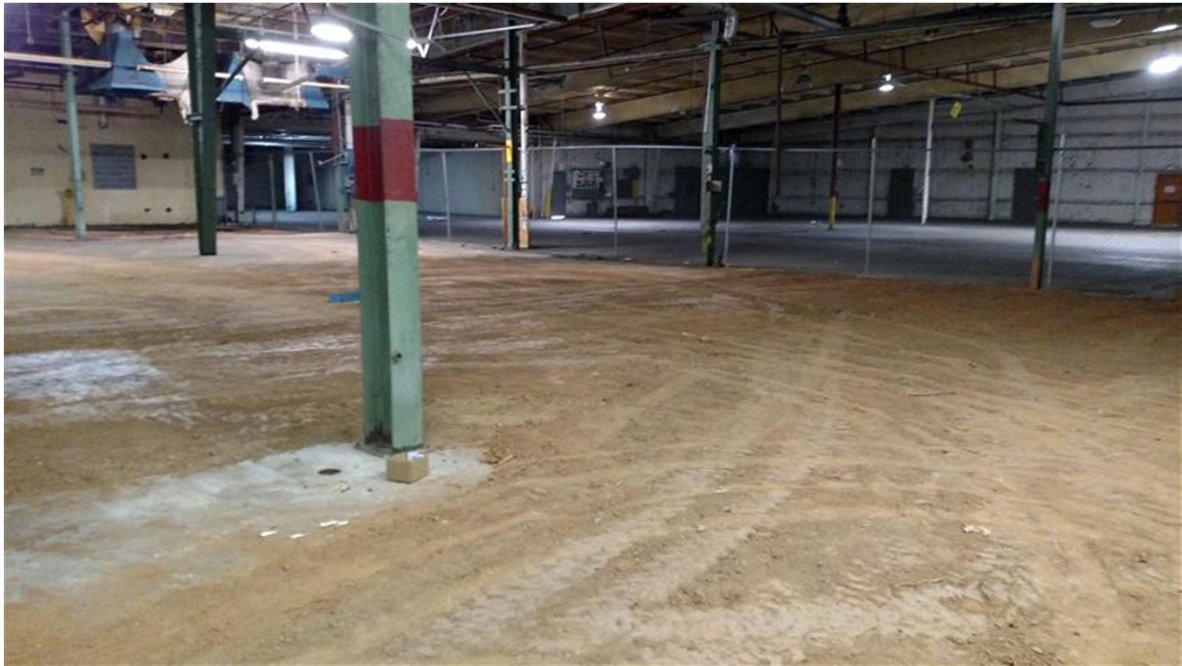
21. Production area with large floor drains filled with dirt.
