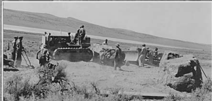
Dragging 20 ton boulders for the "Portal" pictured on background of this page.
