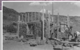
Color picture as it appears today and inset of construction of the Overnight Cabin in August 1937.
