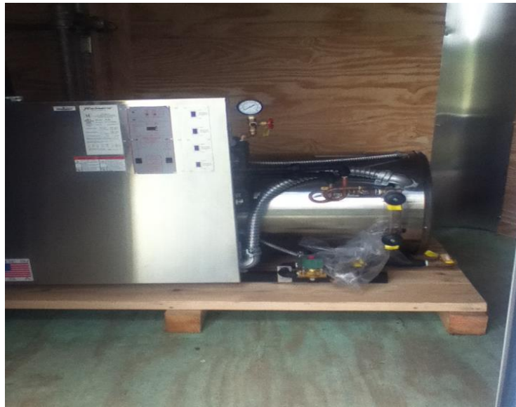
Figure 26. The electric steam boiler is equipped with 100 kw heating elements.
