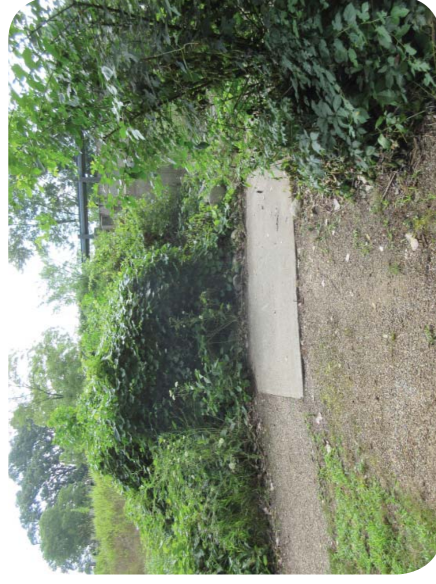
CRUSHED GRAVEL PATH CONNECTION TO CONCRETE SIDEWALK DOES NOT MEET ADA STANDARDS.
