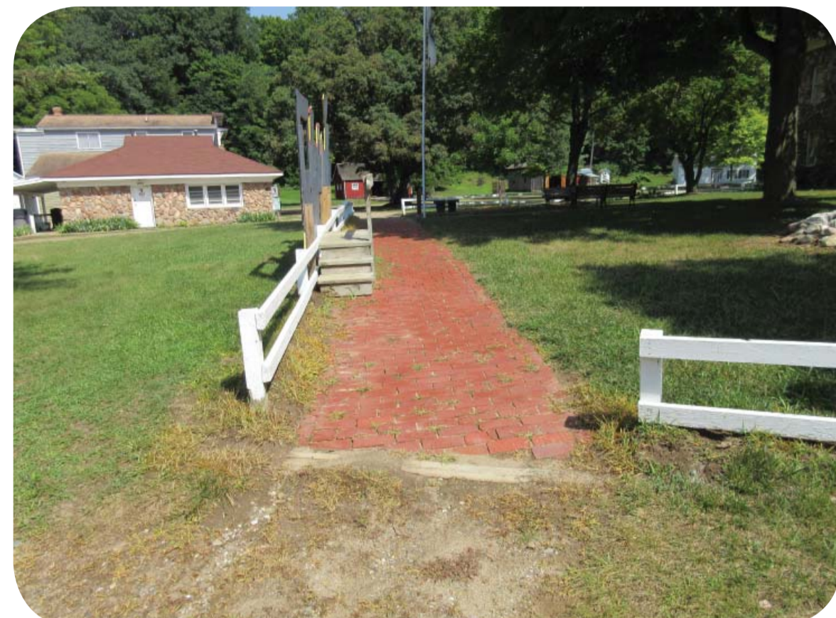
PAVED PEDESTRIAN WALKWAY TO VILLAGE IS NOT ADA ACCESSIBLE.
