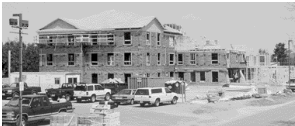
During the winter, spring, and summer of 2001, New Hall was under construction and on its way to becoming the college's eleventh residence hall (above). It was completed (see cover photo) in time to welcome students to the beginning of the school year and has engendered a great deal of positive student response.
