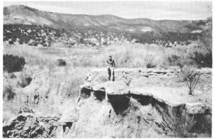
FIGURE 1.6. East abutment, old US-70 highway bridge in 1991, at Bent. This part of the road was abandoned about 1936 and the erosion visible here has occurred since that time. (Photograph by Paul Bauer)
