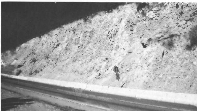
FIGURE 1.24. Leached collapse breccias in San Andres Formation west of Cloudcroft at mile 66.0. Slumping of these materials in roadcuts causes problems for the Highway Department.
