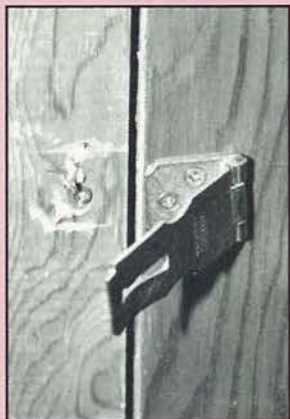
The hasp on the laundry storage room was damaged with a broken towel bar. Photo by Rick Wiedmaier.
