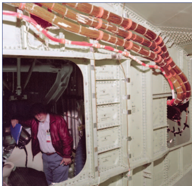
Figure 4.2-3. Typical wiring bundle inside Orbiter wing.
