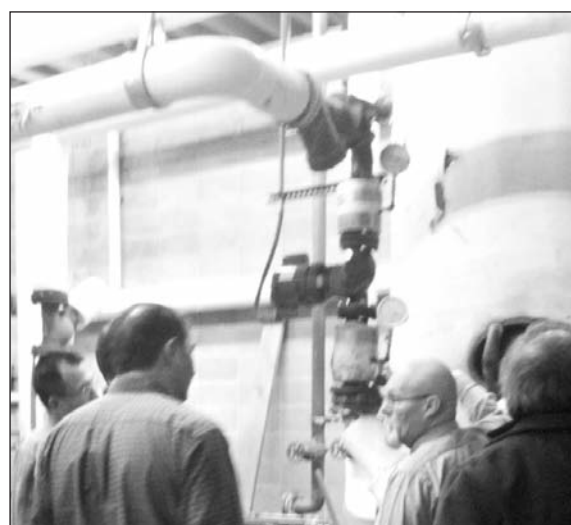
Matt McClain, FUSD Energy Conservation Supervisor, points out some of the deficiencies of the current American High School HVAC system
