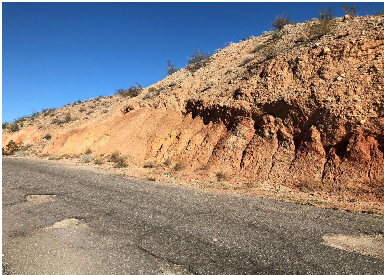
Figure 13. Damaged Pavement in Zone 1
