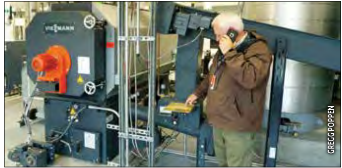
Biomass-fueled heating gear at the airport displaced an old diesel-fired system.
