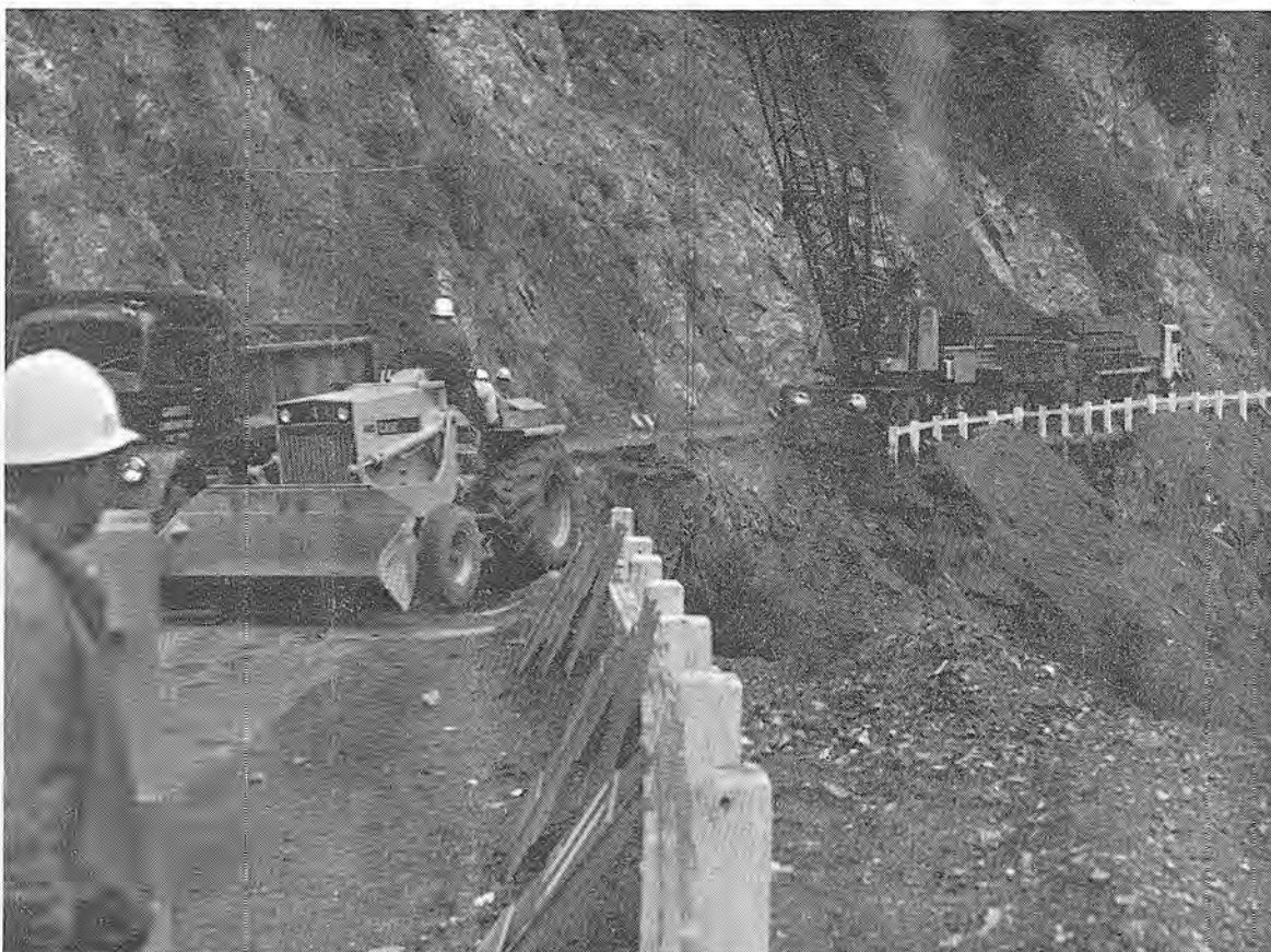
SLIP-OUT ON 101 above Cummings caused by heavy rains and resulting slide conditions is put back in shape by Granite Construction Co. At left Super Tap Fausey watches Brother Rowland operate the loader while further along Brother Turley and his son operate the clam shell.
