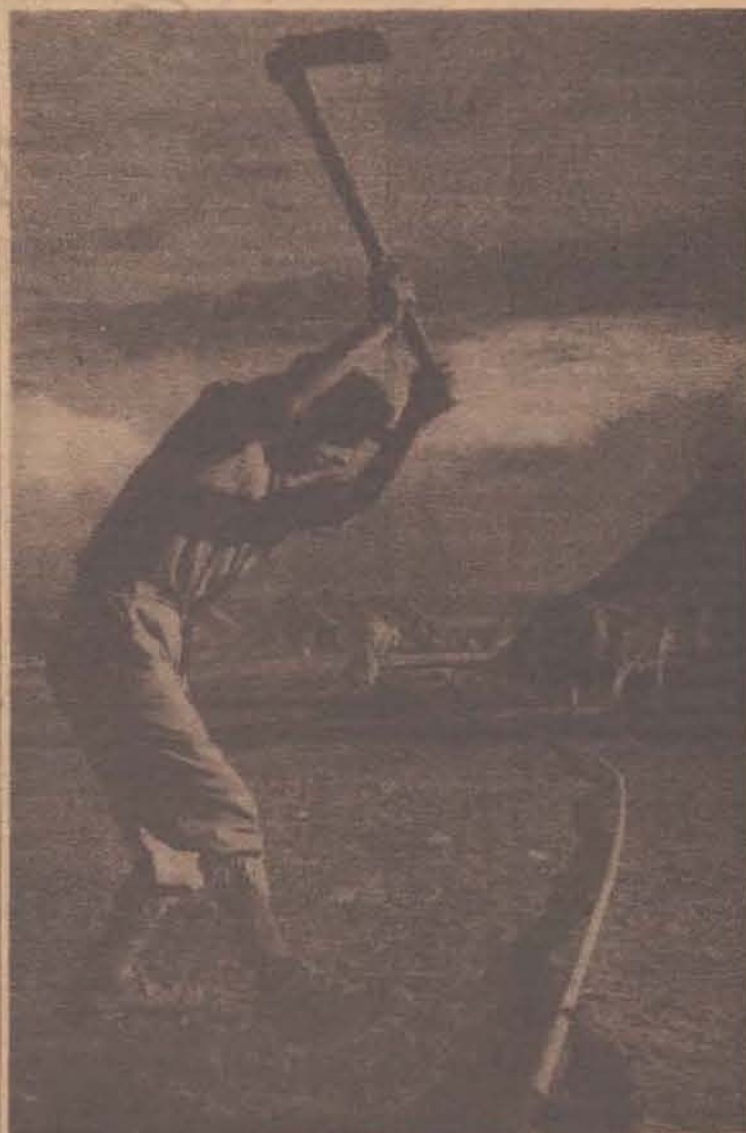
EVERYONE TOILS IN THE NEW ISRAEL. Worker wields pick to bury newly laid water pipe.
