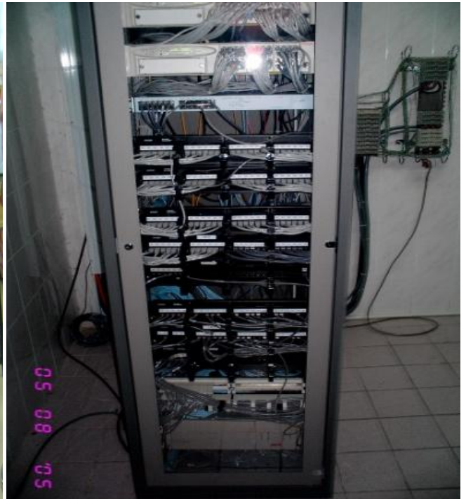
Central Wiring Room – UMP Pekan
