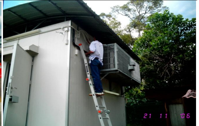
Cop System – Celcom Eastern Region
