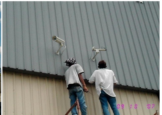
CCTV System – Telekom Cheras
