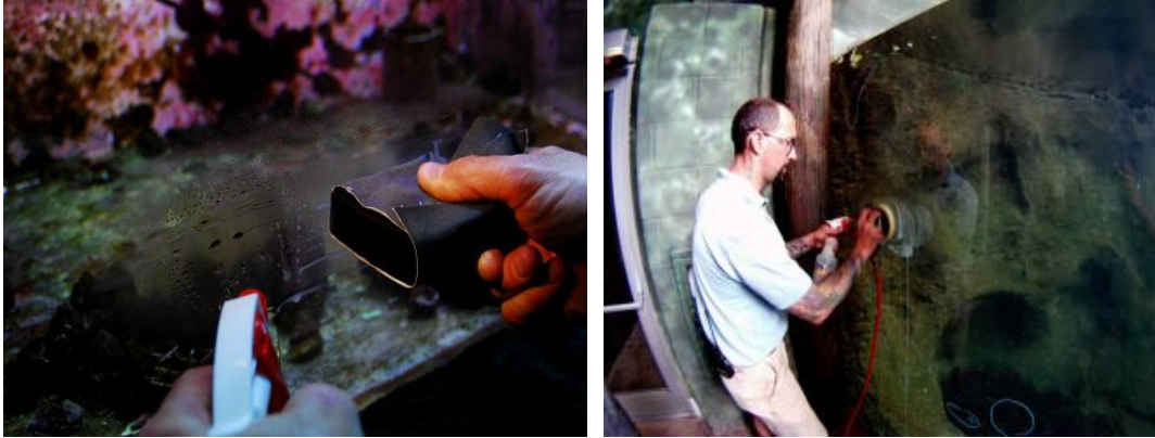
Figures B and C: Spray water on dry-side work areas while buffing.
