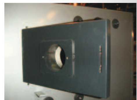
Oil burner hatch
