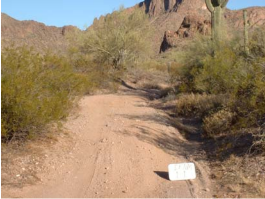
1-1 erosion after wash
