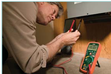
CAT IV application measuring voltage on a 480V 3-phase transformer
