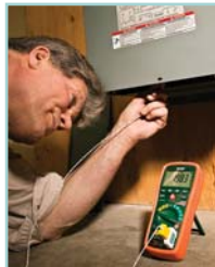
Measuring the internal temperature on a 3-phase transformer installation
