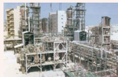
After the completion of stage expansion, SHARQ has the capacity to produce 2.5 million tons of ethylene, 1.4 million tons of polyethylene, and 1.55 million tons of ethylene glycol per year, almost double the existing capacity. SHARQ thus has the largest annual production capacity for a single plant in the world.
