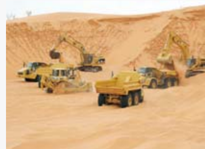
Construction equipment leased by AJIL is contributing considerably to Saudi Arabia's advancement in fields such as domestic infrastructure development and urban development.
