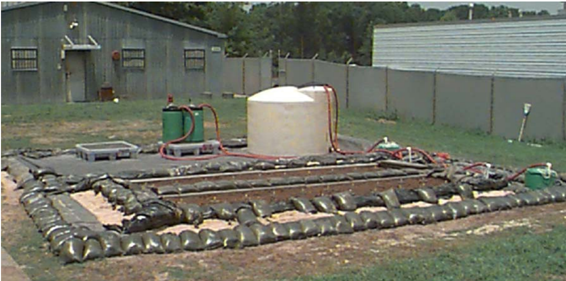
Figure 11. Photograph of the LTU pilot project illustrating the land treatment units, the primary and secondary containment systems, and the leachate collection system
