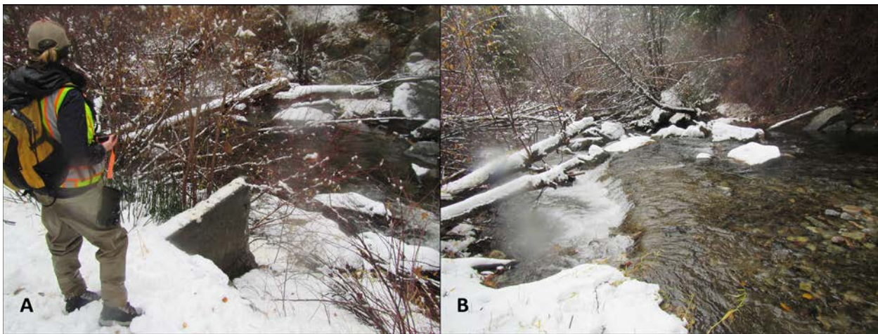
Figure 35. A) cement wall on bank at RM 1.42; B) cement slab on channel bed at RM 1.33. (Photos: IFI 11/9/2017)
