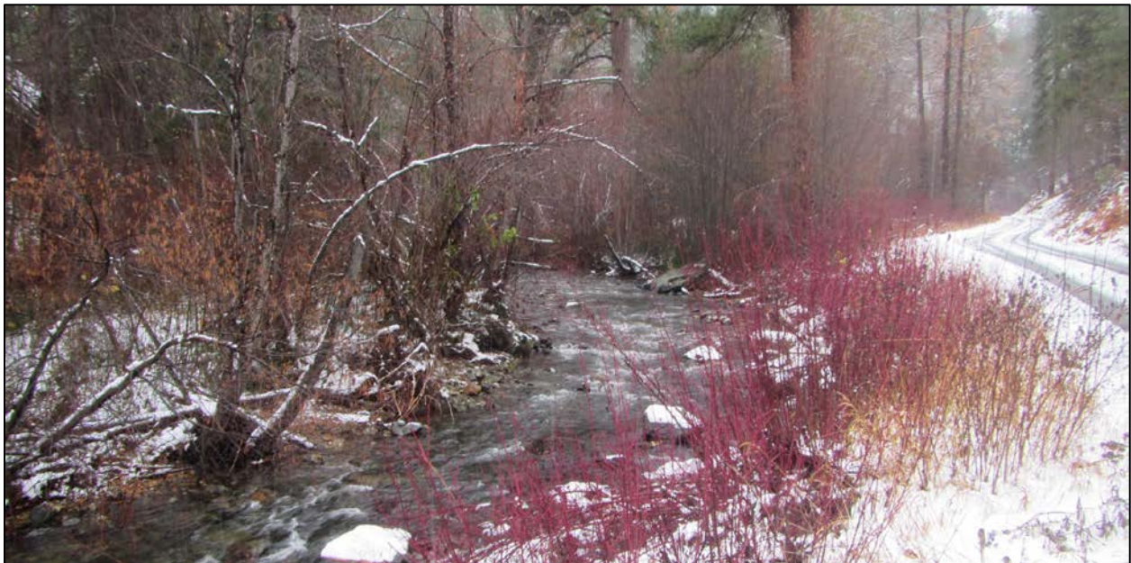
Figure 46. Mad River Road occupying valley floor and the associated impaired riprapped channel bank. (Photo: IFI 4/9/2017)
