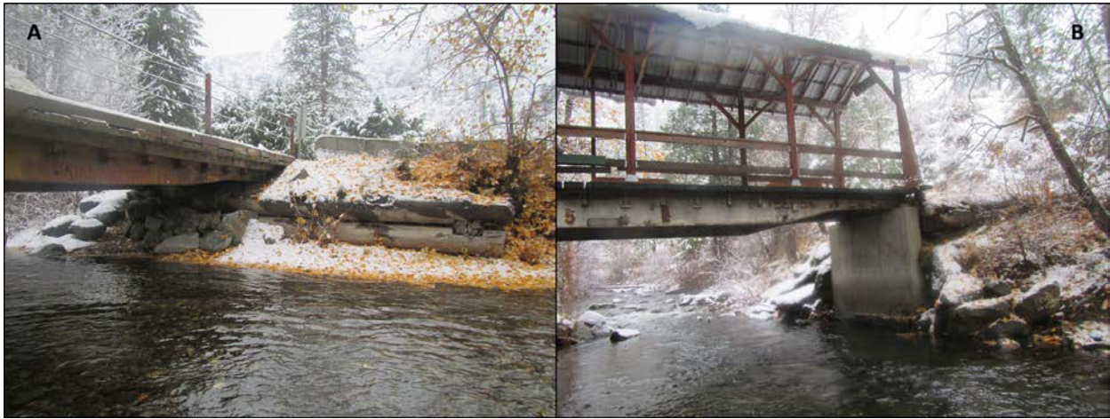
Figure 24. Railroad-car bridge crossings: A) near RM 0.3 with log, cement, and riprap footings and bank protection. Logs are old footings from historical bridge crossing, and B) near RM 0.6 with cement footings and large boulder riprap. (Photos: IFI 11/9/2017)
