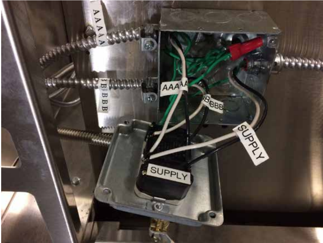
MAIN ELECTRICAL BOX SHOWING SUPPLY LINE ENTERING ON RIGHT SIDE OF BOX.
