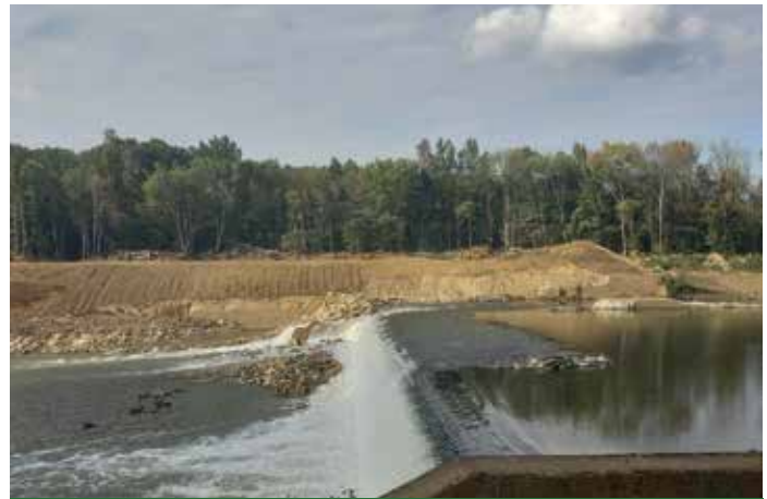
Workers removed Lock and Dam 5 on Green River in the summer of 2022. The removal of Locks and Dams 5 and 6 frees 73 miles of formerly impounded water on the Green River. Photo: Eric Cummins
