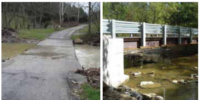
In a partnership with Harrison County Fiscal Court, a new bridge crossing was constructed across West Creek. This improvement allows fish and mussel passage into the upstream reaches of West Creek. Photo: KDFWR
