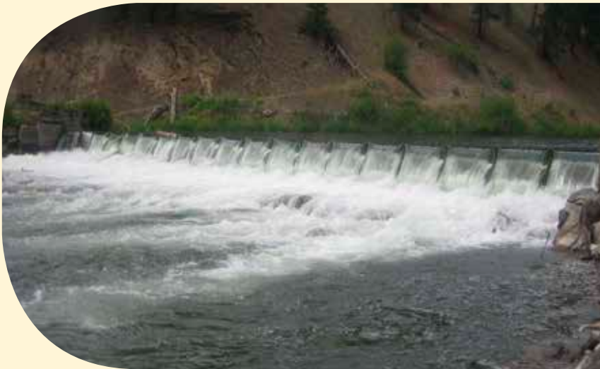
French-Grass Valley Diversion Dam on the Clark Fork just west of Missoula - diversion dams can be dangerous when flash boards are installed, creating a large drop and unpredictable conditions below.
