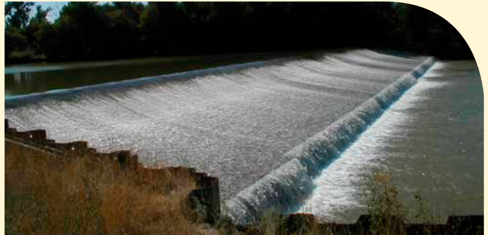
Tongue & Yellowstone low head diversion dam on the Tongue River at low flows.
