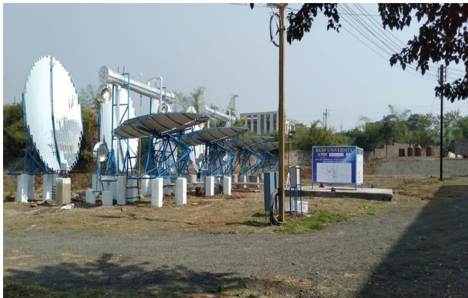
Figure 15- Solar-powered Scheffler Dish steam generation system at RKDF University (MNRE funded project)
