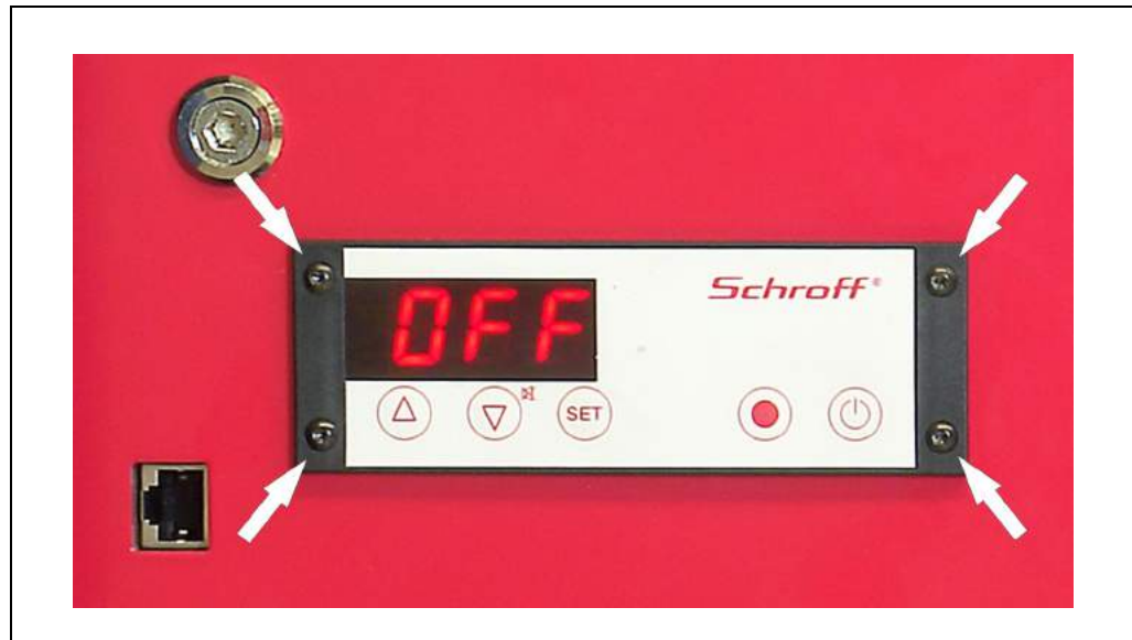
Figure 7: Control and display unit
