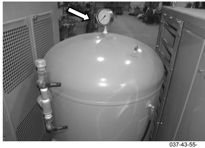
Figure 36: Compressed Air Pressure Gauge –Tank mounted on TYPE II Control/Distribution Center
