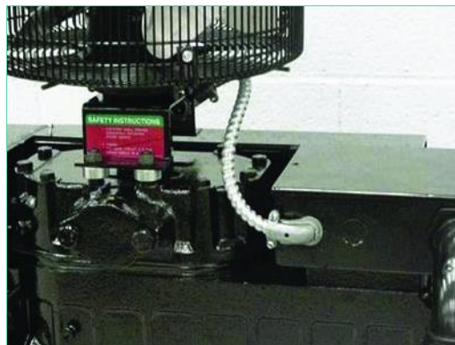
Figure 2.4 3D Fan Installation
