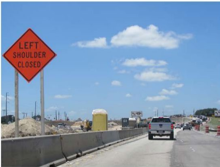
MoPac Intersection Project work continues at Slaughter Lane. (Nicholas Cicale/Community Impact Newspaper)
