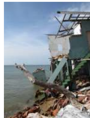
Loss of property due to coastal erosion in Trinidad Photo courtesy Robyn Cross
