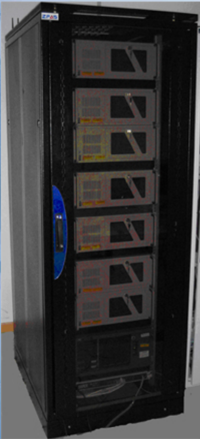
Rack mounted Probes
