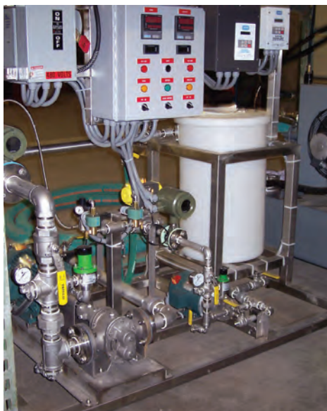
Utilizing ECO GA12 Flanged Pump to pump resin.
