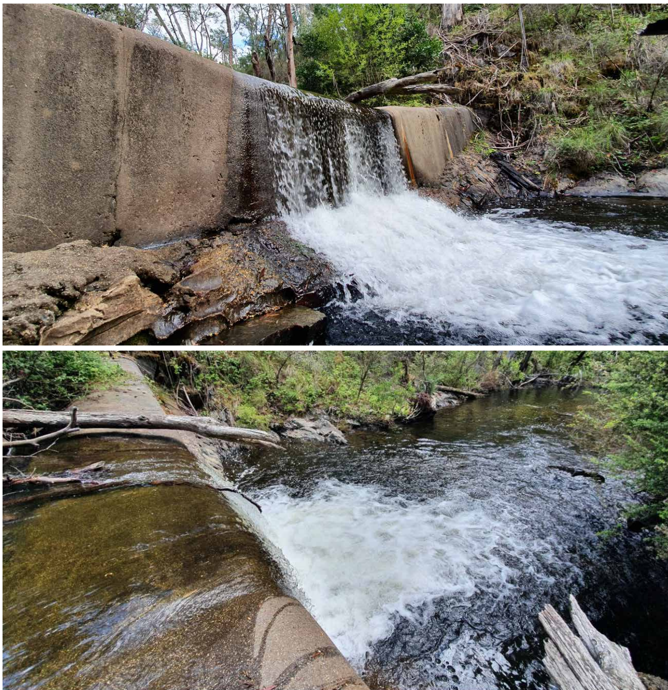
Figure 1. The concrete barrier to prevent upstream fish movement within the Big River catchment, Victoria; (top) looking at the face of the barrier, and (bottom) from the barrier looking downstream. Images: Matt West.
