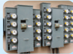
Energy Management System
