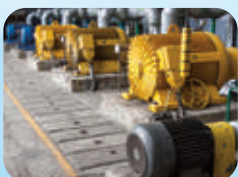
Pump Station Management
