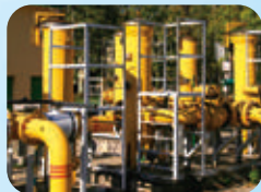
Storage Tank Monitoring
