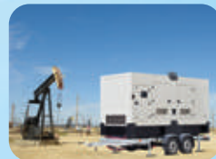
Outdoor Generator Monitoring
