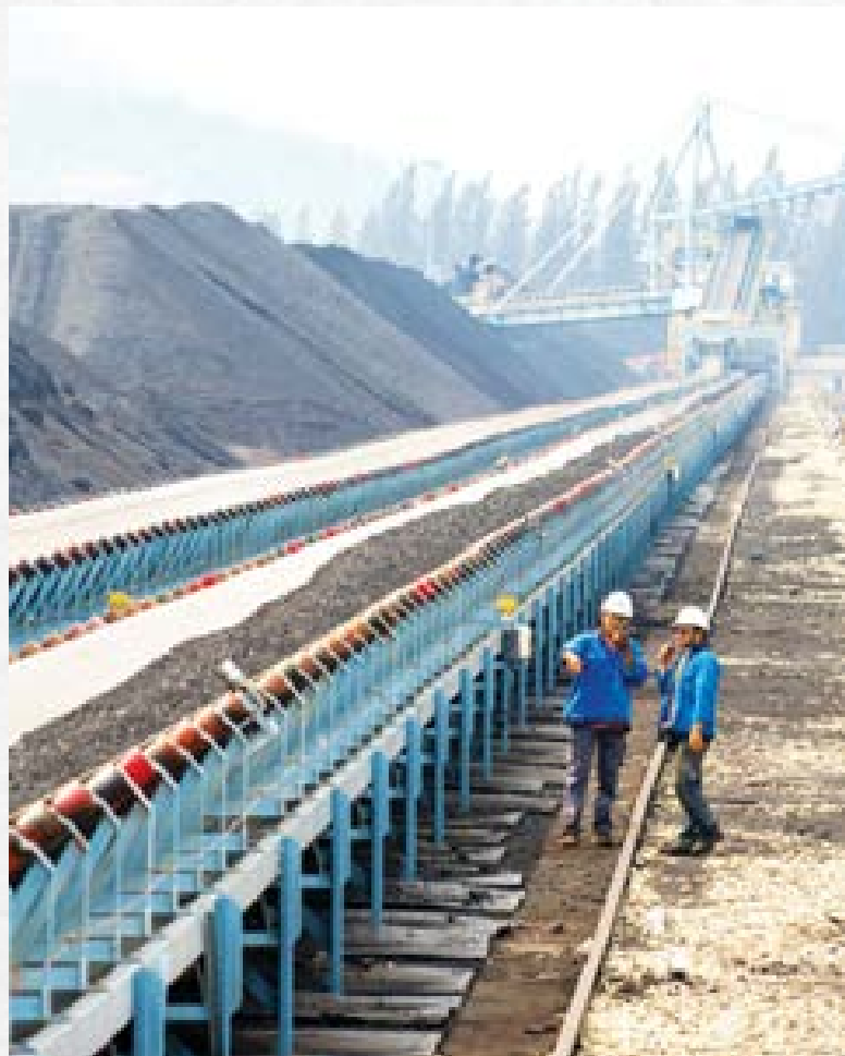
Staff monitoring the daily operations at the Sultan Azlan Shah Power Station, Manjung, Perak.
