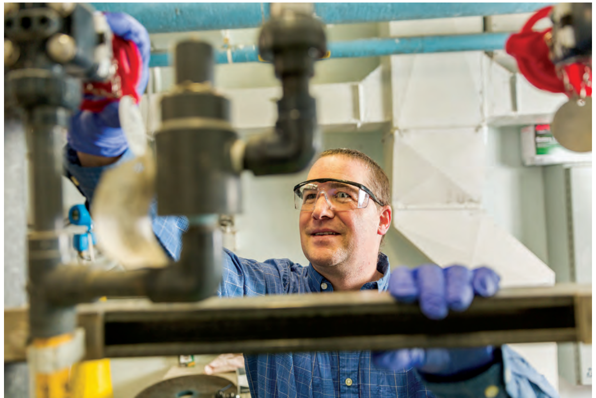
Timothy King tests for chlorine residual (upper photo) while Dan Driscoll swaps a chlorine pump as part of a regular rotation.
