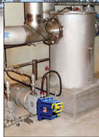
Condensate/Sediment Trap with Electrically Actuated and Manual Drip Traps
