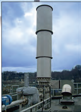
Enclosed Waste Gas Burners
