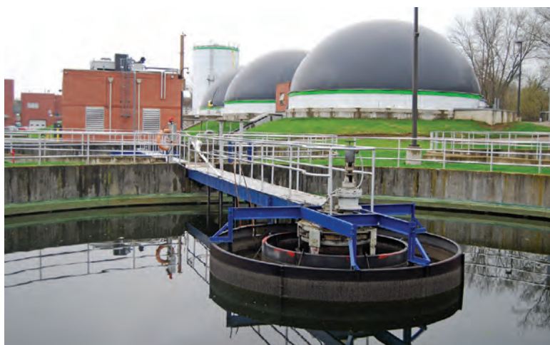
The three upgraded anaerobic digesters sit behind one of the Wooster plant's final clarifiers.
