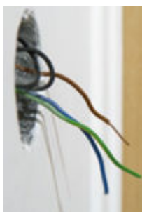
Exposed electrical wires.
