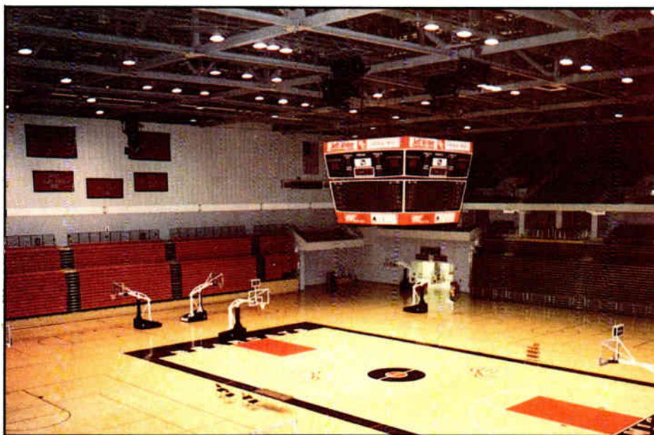
The arena system is composed of eleven speaker clusters which are selectable at the equipment rack.
