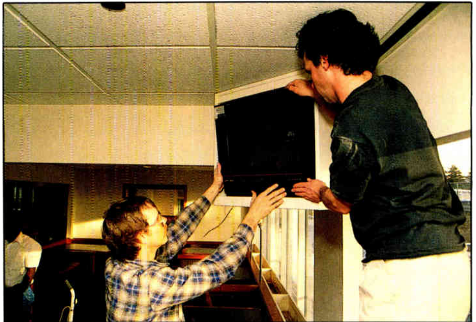
A series of Zenith 20-inch monitors were installed around the room.
